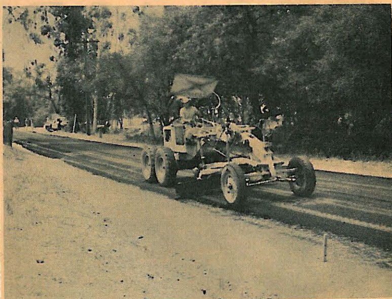
County Highway motor patrol spreading oil mix surfacing on Arnold Way east of Tavern Road. Echo Photo.
